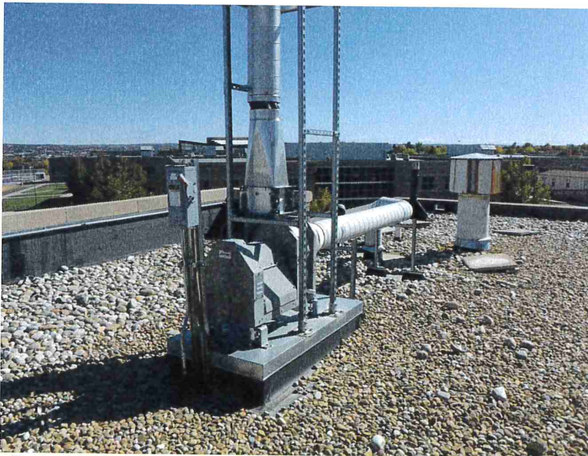
Photo 12 – Roof equipment was mounted on curbs, similar to the exhaust fan depicted. There were no observed holes or tears in the membrane at the curbs.
