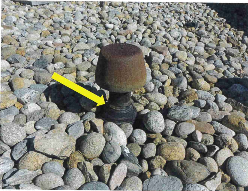
Photo 11 – Roof penetrations had flashing boots and clamp rings (indicated) at most locations.
