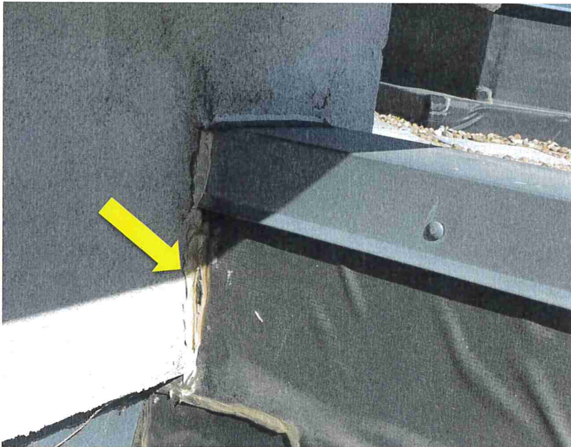
Photo 19 – Multiple layers of sealant were visible at the EPDM to EIFS transition at the southwest section of the ballasted EPDM roof.
