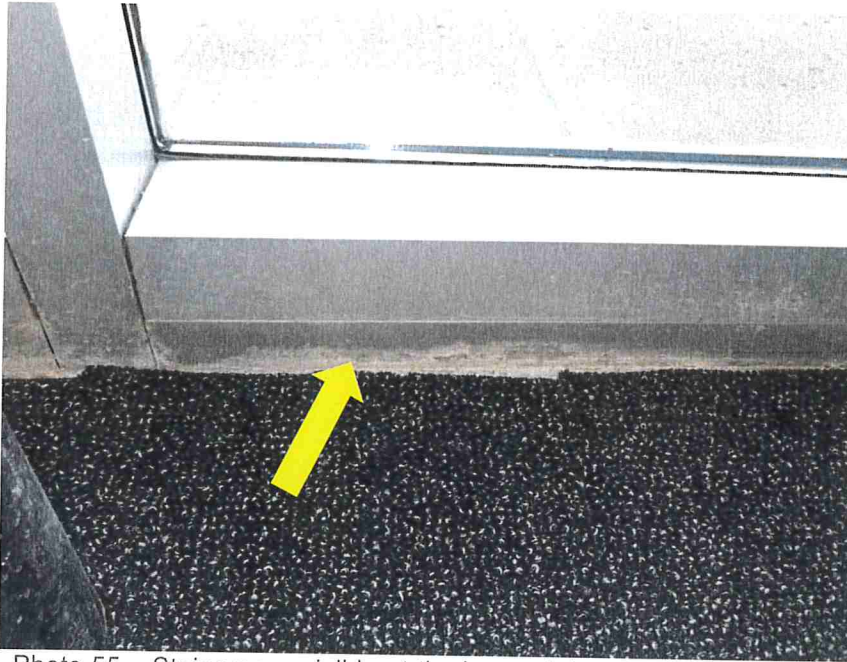
Photo 55 – Stains were visible at the base of the entrances, along the interior.
