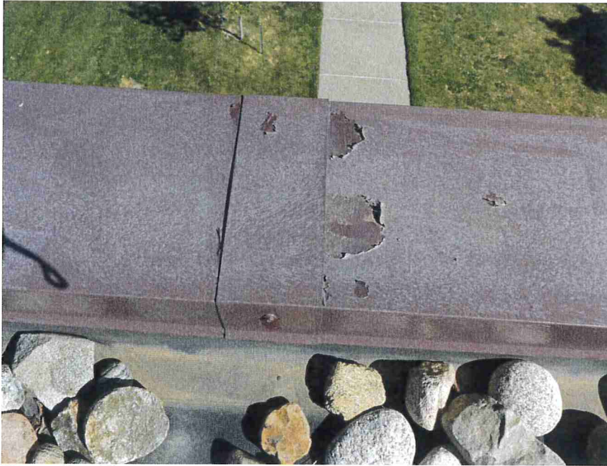
Photo 27 – The paint on the metal coping was peeling.
