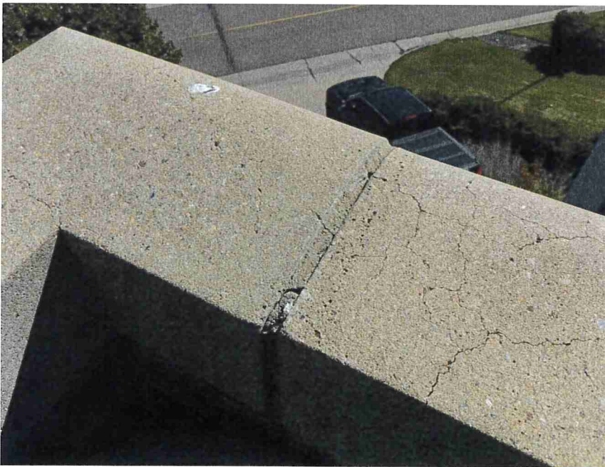
Photo 16 – Precast coping and mortar joints at the top of the parapet had cracks.
