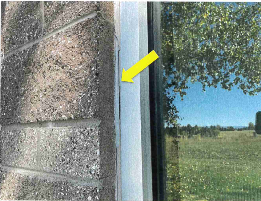
Photo 50 – Sealant was missing at a portion of the window jamb, but the remaining sealant did not have cracks or holes.
