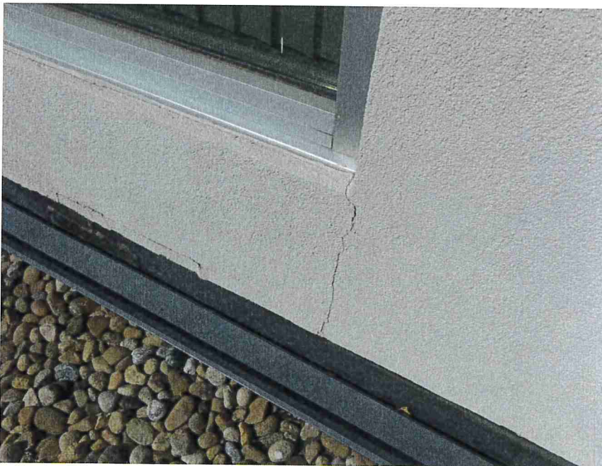
Photo 36 – A crack was located at the bottom corner of the window opening in the EIFS on the north wall.
