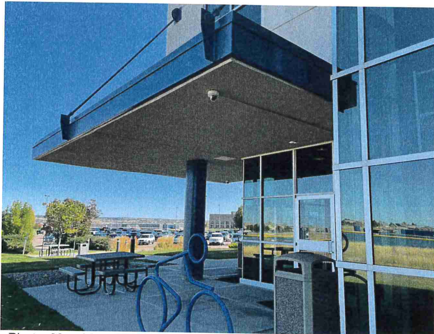
Photo 60 – View of the canopy soffit at the northeast corner of the building. No cracks or staining were observed at this location.
