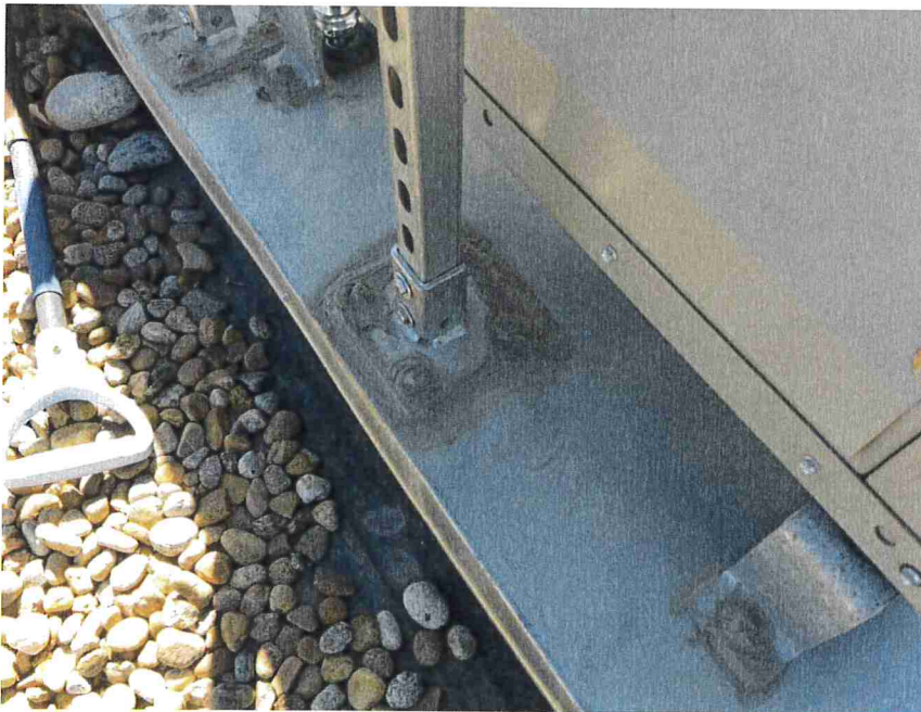
Photo 14 – Sealant was placed around fasteners at the exhaust fan. No holes were observed in the sealant.
