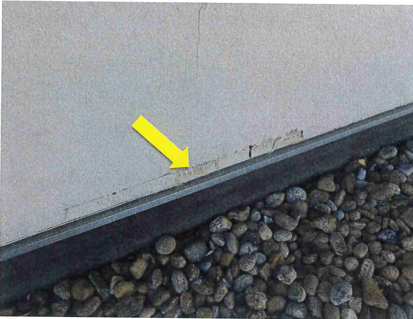
Photo 35 – Along the west EIFS wall, the mesh was visible at the base of the wall.
