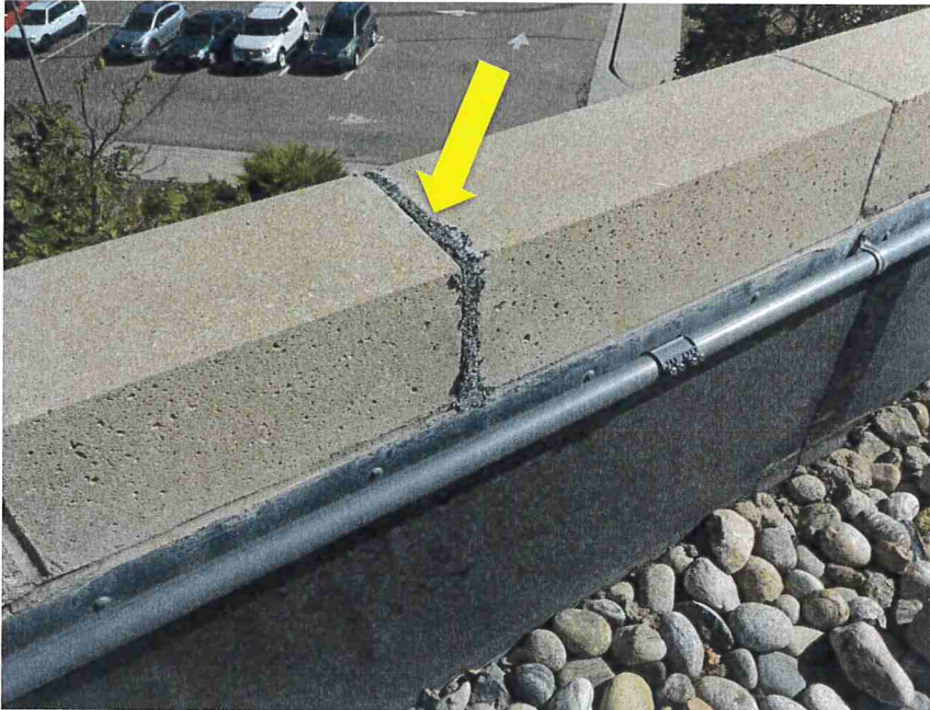
Photo 17 – Mortar at the joint between sections of precast coping appeared different from adjacent areas.
