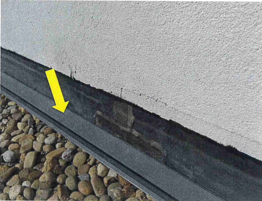
Photo 23 – Flashing was not secured below the EIFS on the north side of the main roof area. A section of flashing was resting on the roof.
