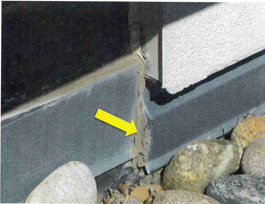
Photo 24 – Flashing was placed directly above the membrane, and the membrane did not extend 8-inches up the wall. Sealant joints were placed at the ends of the flashing (indicated).
