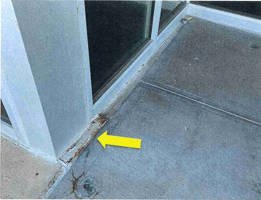
Photo 53 – A steel base plate was exposed and corroded (indicated) at the exterior of the storefront at the north entrance.
