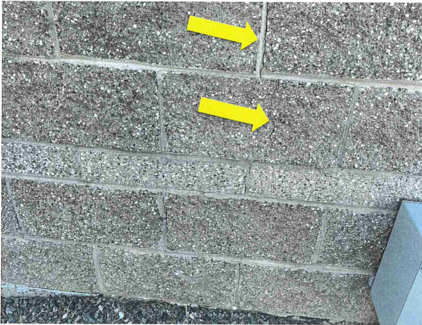
Photo 45 – Cracks in the exterior were observed at the southeast corner (indicated). The cracks were in the mortar joint and across the split-face CMU.
