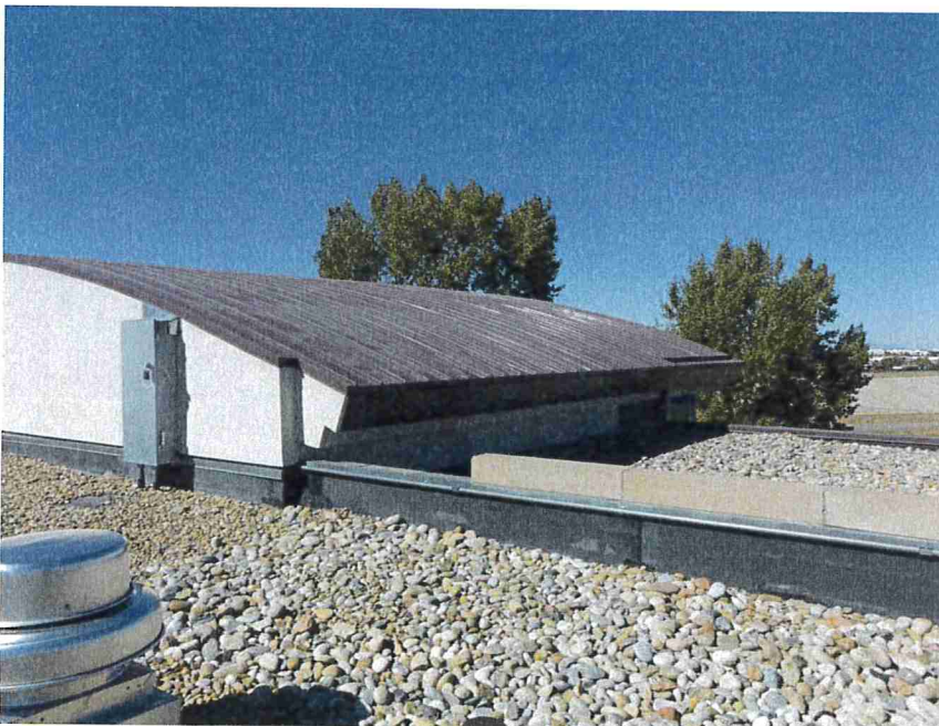
Photo 30 – View of the curved profile at the standing seam metal roof at the northwest corner of the building.
