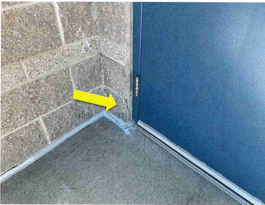
Photo 46 – At the southeast corner of the building, the face of the CMU was cracked at the door jamb.
