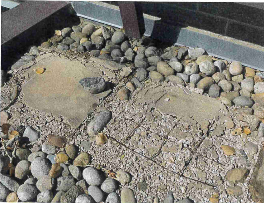
Photo 29 – Pavers were crumbled with exposed aggregate and reinforcement.
