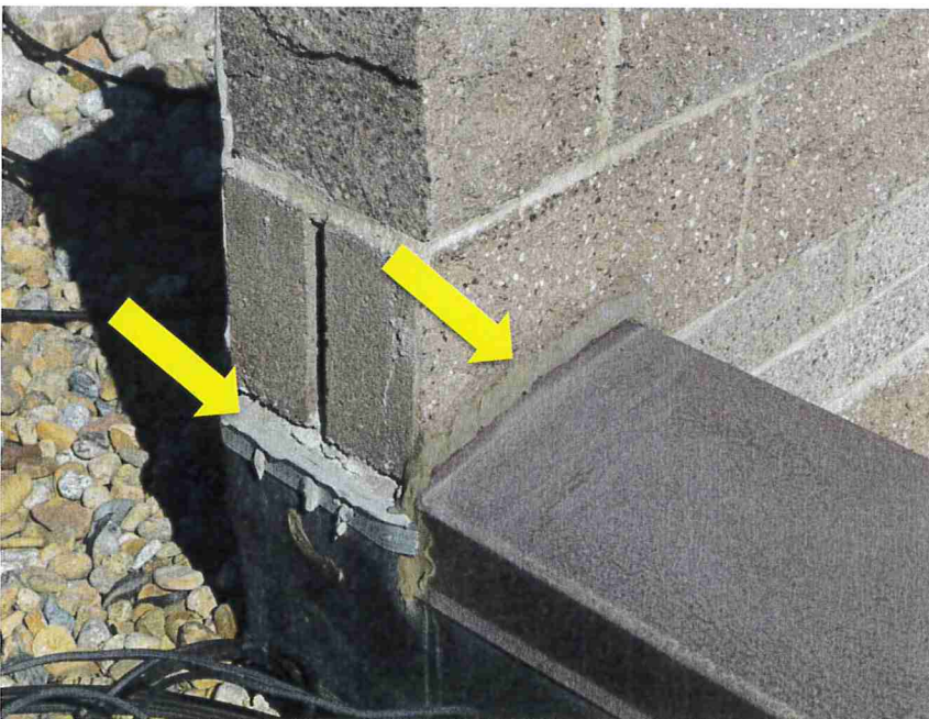
Photo 20 – Sealant joints were placed at the top of the exposed termination bar and at the metal coping to wall transition.
