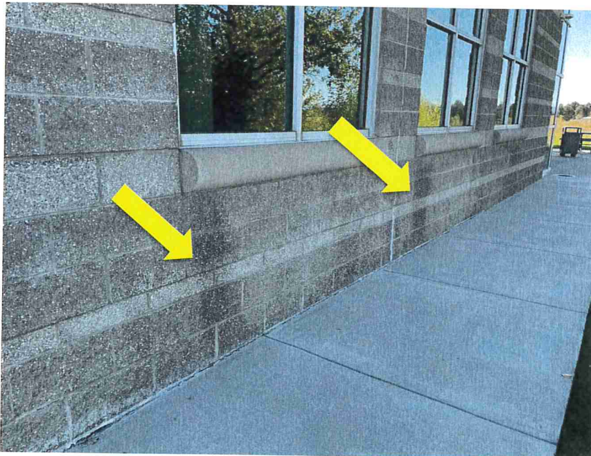
Photo 44 – Discoloration was located below the windows on the first level.
