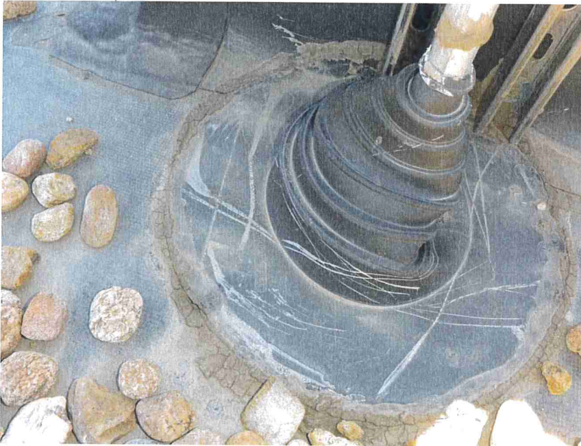
Photo 13 – Sealant around the membrane flashing was cracked and brittle, although was still bonded to the membrane.
