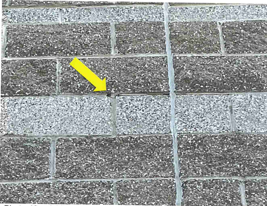
Photo 43 – Additional weep holes were observed around the building exterior.
