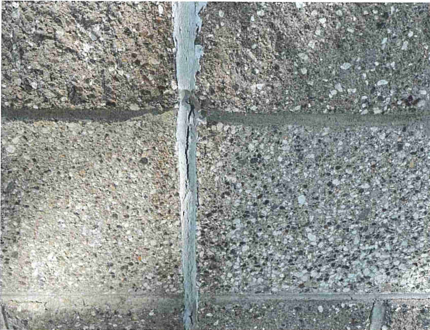
Photo 41 – Sealant at some control joints had holes and gaps, allowing water and moisture to enter the wall assembly.
