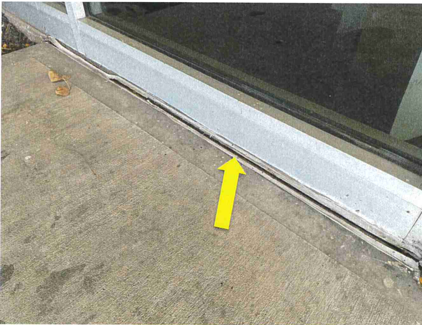
Photo 52 – Cracks and holes (indicated) in the sealant below the storefront system were observed around the building perimeter.
