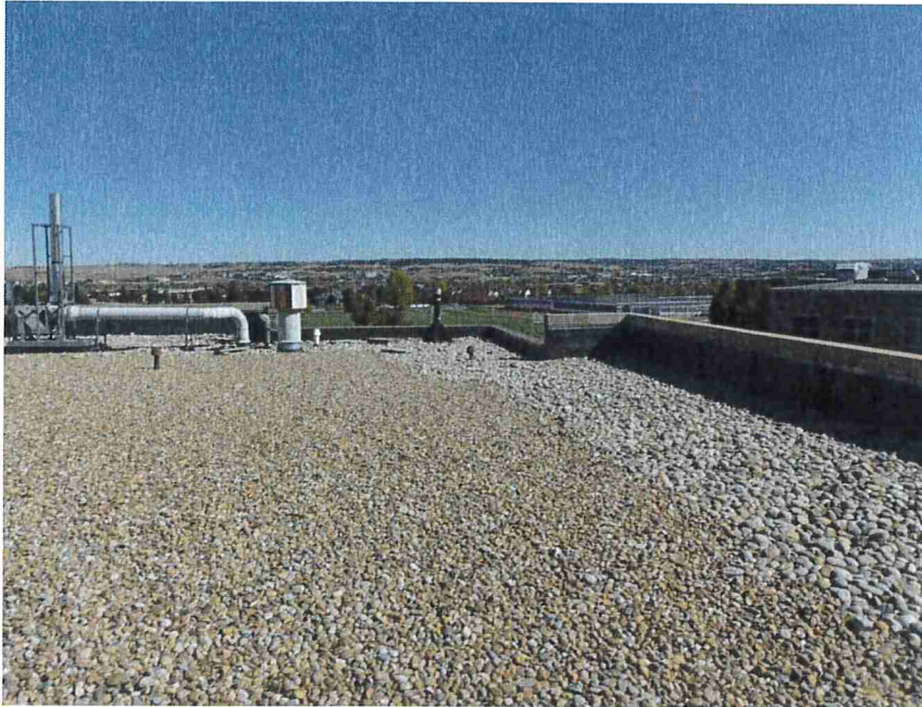
Photo 7 – Overview of the south roof area with a ballasted EPDM system , facing east.
