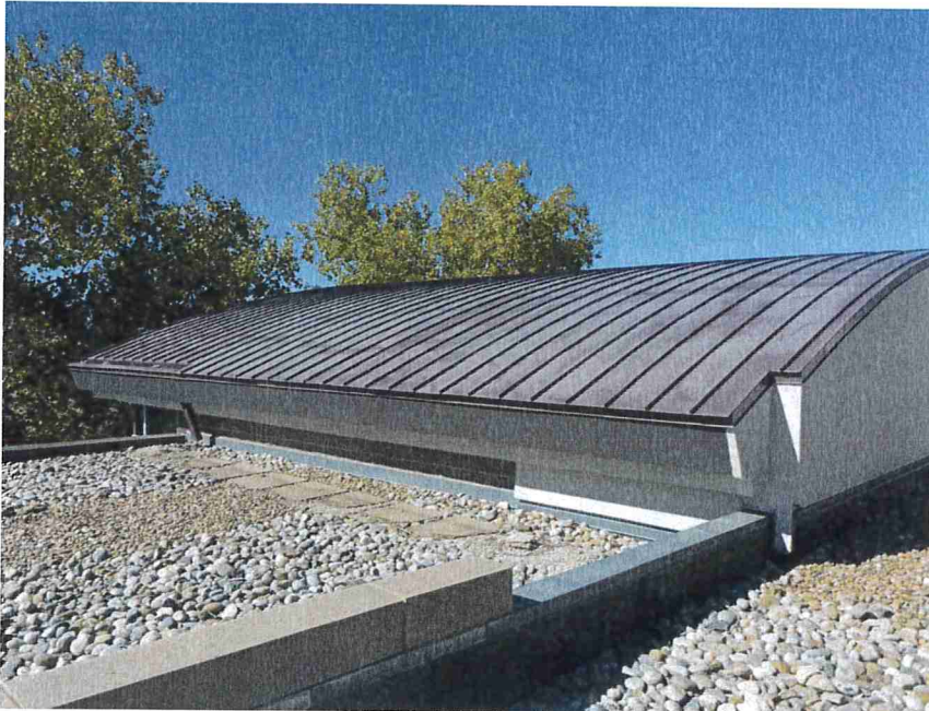
Photo 31 – View of the standing seam metal roof at the west side of the building.
