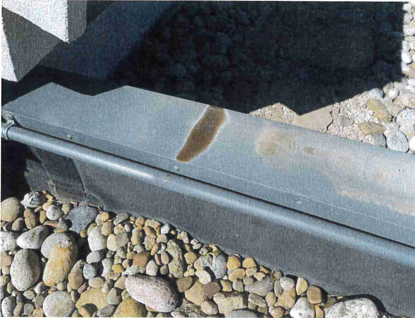
Photo 25 – Coping was corroded at the parapet wall between the main and northeast ballasted EPDM areas.
