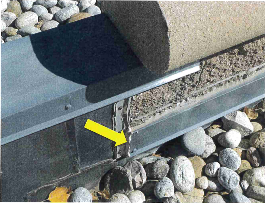
Photo 21 – Sealant was placed at the ends of roof flashings. The membrane did not extend 8-inches up the parapet wall.
