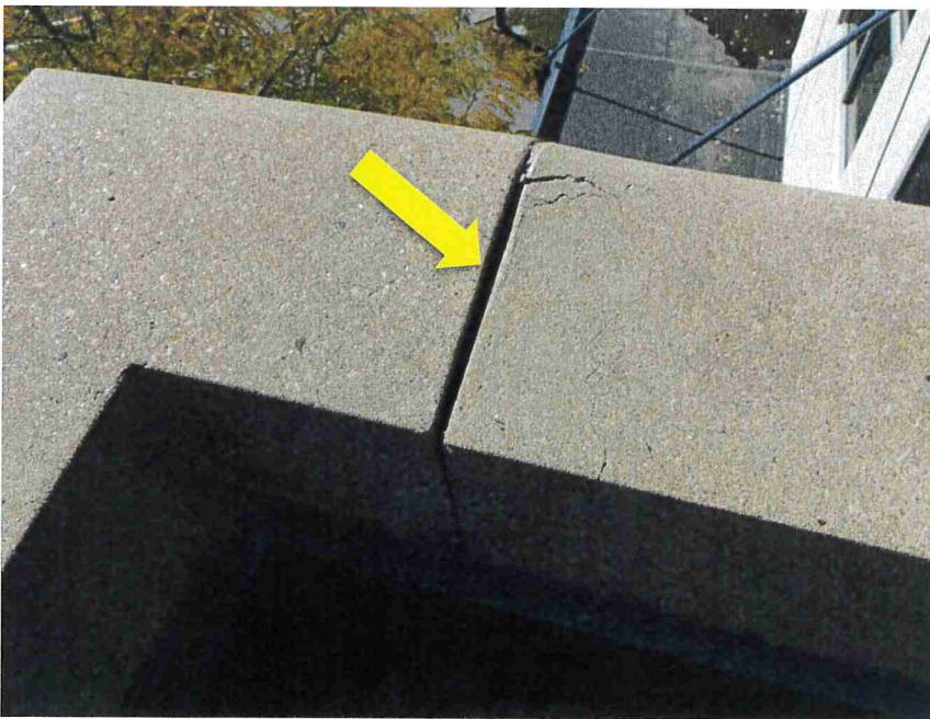
Photo 18 – At the southwest corner of the main roof, the mortar was missing in the joint of the precast coping.
