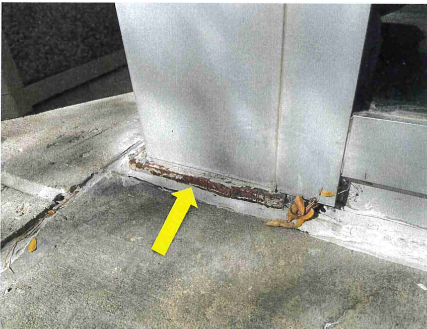
Photo 54 - A steel base plate was exposed and corroded (indicated) at the exterior of the storefront at the south main entrance.
