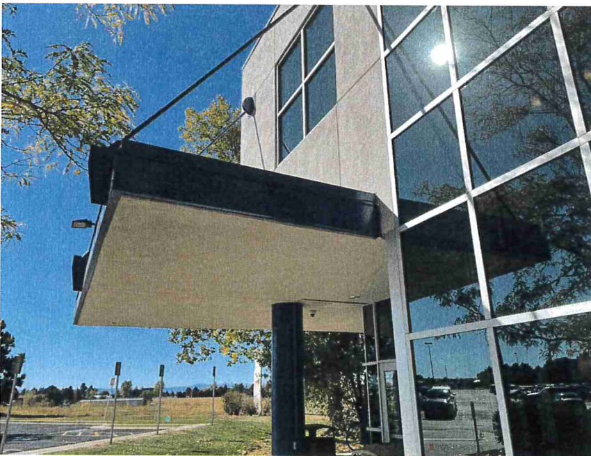
Photo 58 – View of the canopy soffit at the main entrance on the south side of the building.
