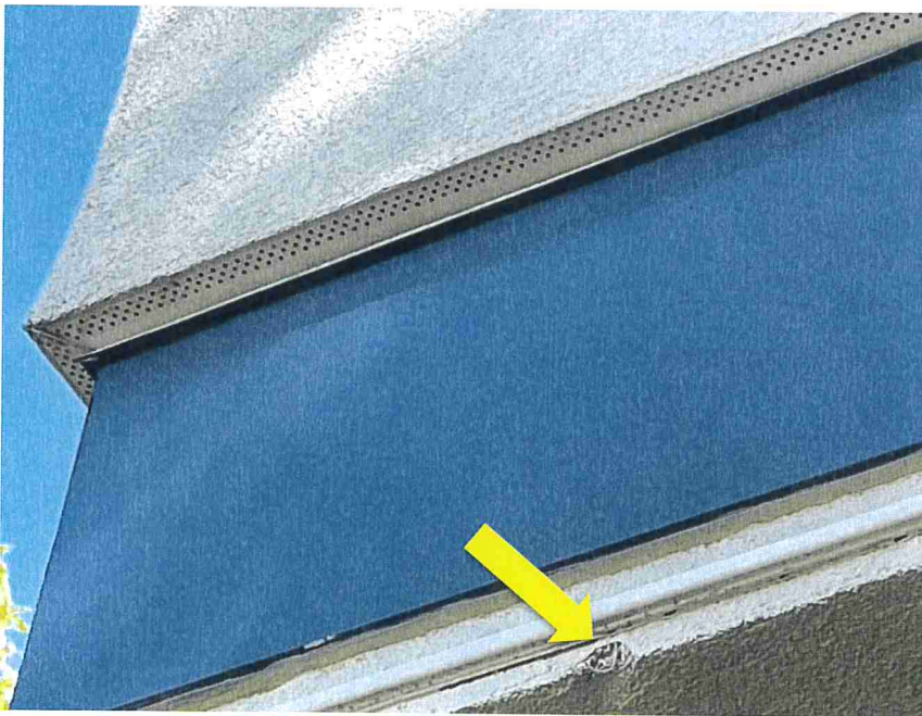
Photo 38 – Weeps were visible below the EIFS on the building exterior. Localized damage to the finish was observed (indicated).
