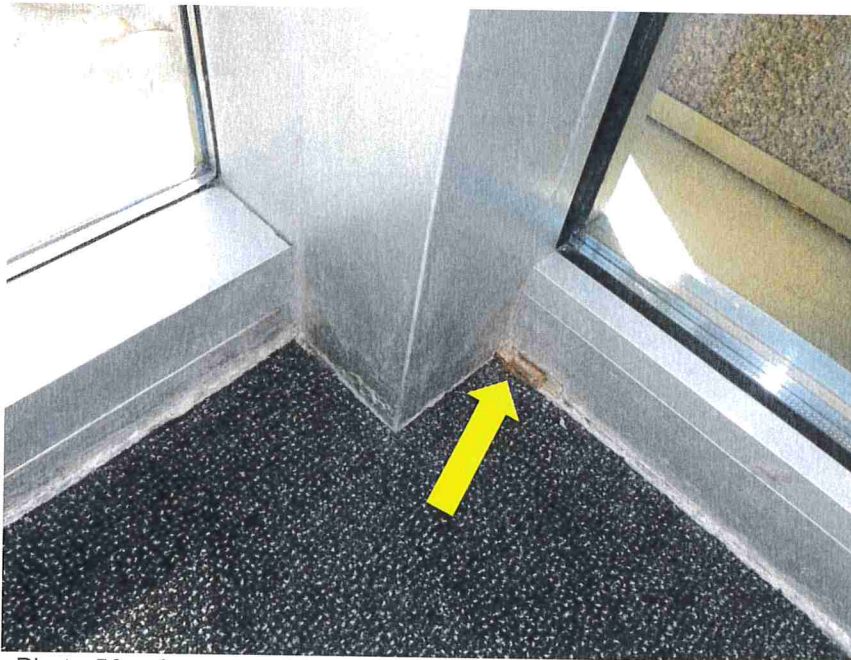
Photo 56 – A corner of the corroded base plate (indicated) was visible from the interior of the building.
