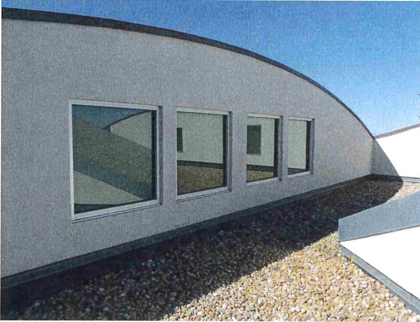
Photo 33 – View of the EIFS exterior along the west side of the main roof area.
