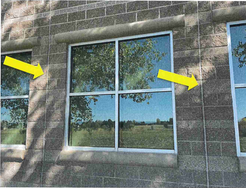
Photo 39 – Control joints were placed in the exterior split-face concrete masonry units (CMU).
