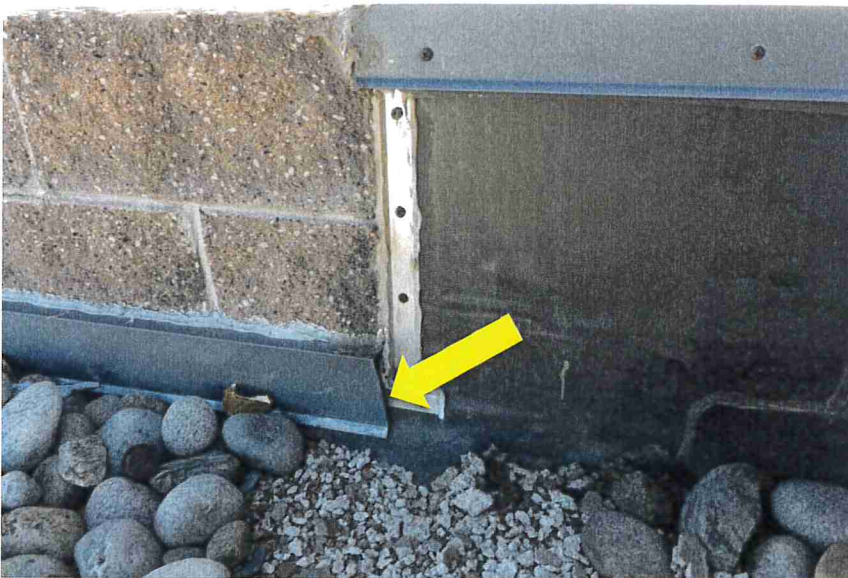
Photo 22 – At the northeast ballasted EPDM roof area, metal counterflashings were placed directly above the membrane. The membrane did not extend 8-inches up the parapet wall. No sealant was placed at the end of the flashing at this location (indicated).
