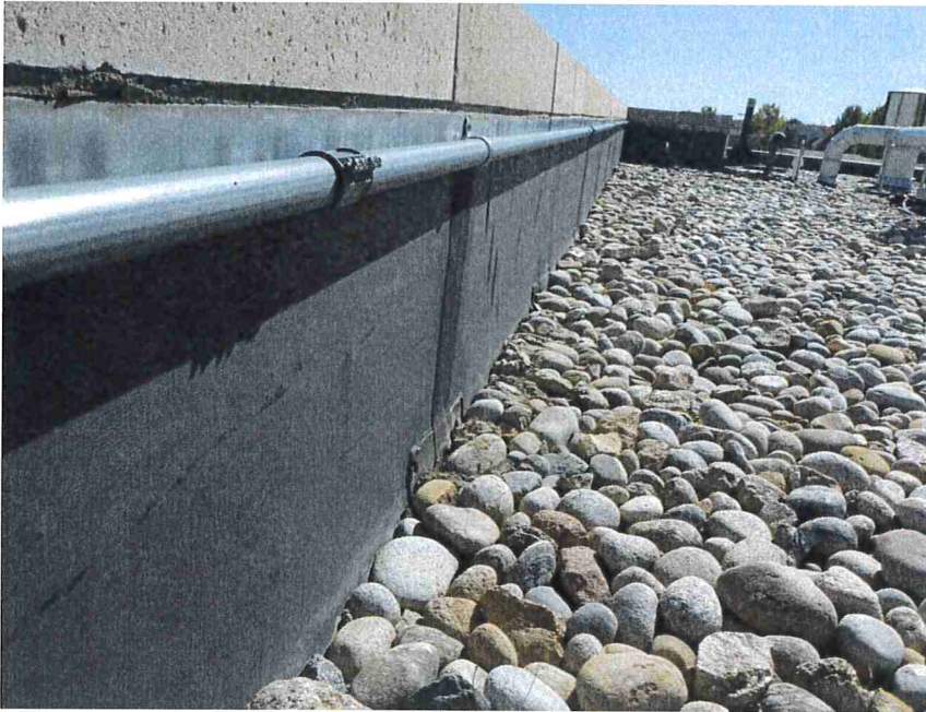
Photo 15 – Along the parapet walls, the membrane was not “tented” or pulled away from the parapet wall.
