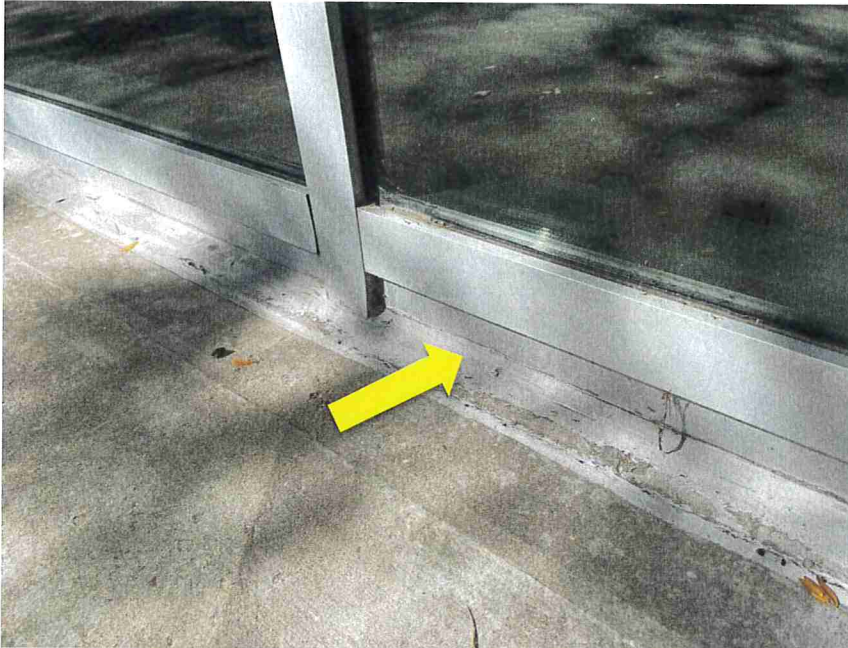
Photo 51 – Sealant joints were located below the storefront systems.
